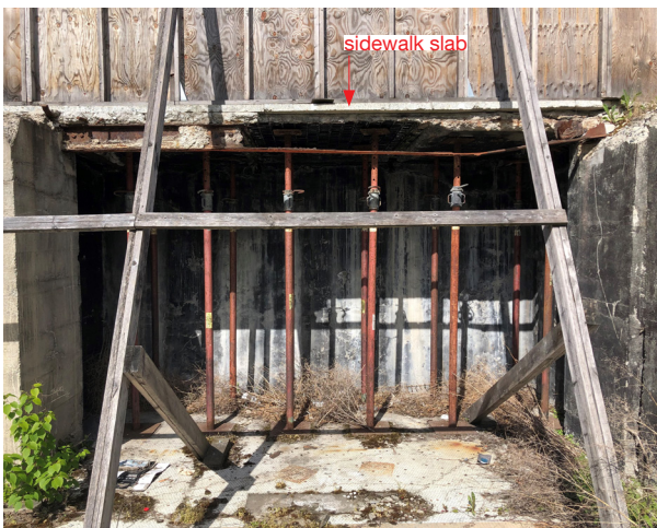
Panel #1 location. All panels are buried under ~4” of sidewalk concrete
