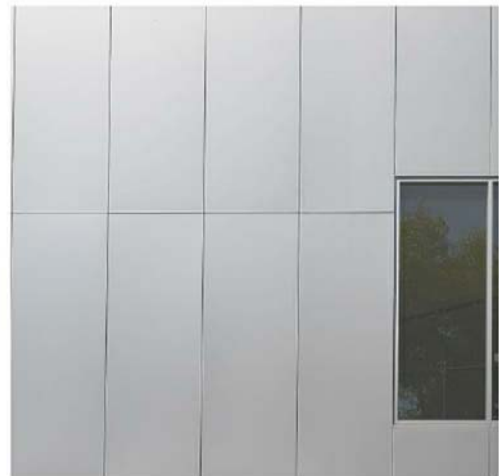
1.1 ▲ COMPOSITE METAL PANEL Residential Exterior
