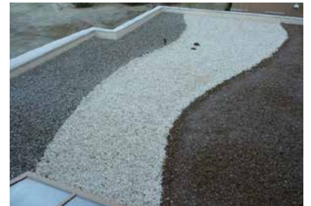
Roof treatment using light and reflective colours to minimize urban heat island effect
