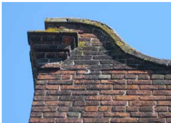
Below: Parapet at rear of Building - no cap flashing noted
