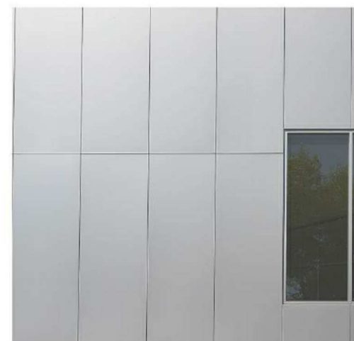
1.1 ▲ COMPOSITE METAL PANEL Residential Exterior
