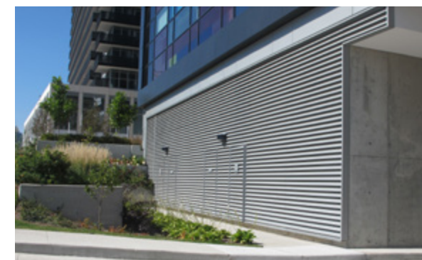
Precedents: Locate equipments in less visited areas and integrate screens into building design.
