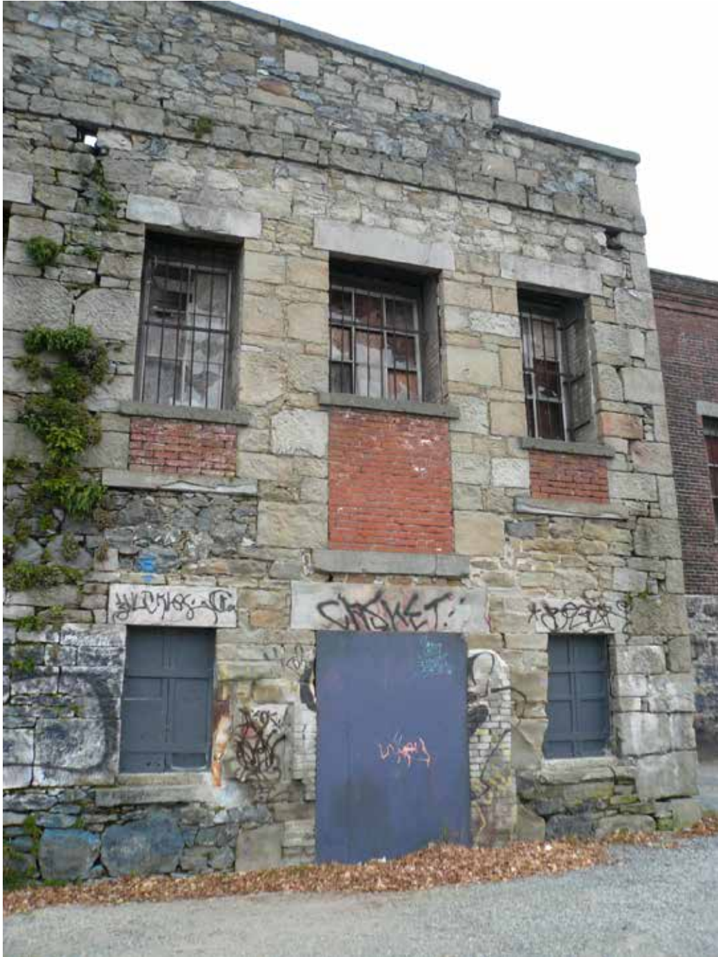
Rear elevation of the Fraser Warehouse showing openings altered using brick, changes to window assemblies, and general condition of masonry.
