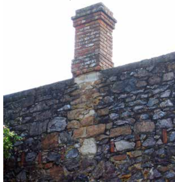
Parapet and chimney at rear of building - no flashings present.
