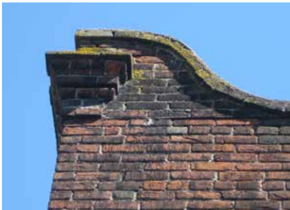
Parapet at rear of Building - no cap flashing noted
